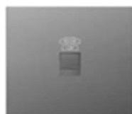
Telephone Socket Outlet
